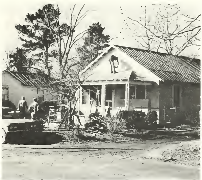
The first house to be repaired under Aurora's CDBG program. Photo by Brian Benson
